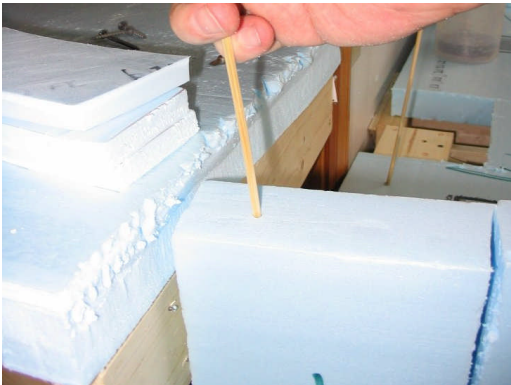
Photo 21 – Force the bamboo skewers through the riser into the foam base. This will hold the riser in place during the rest of construction.
