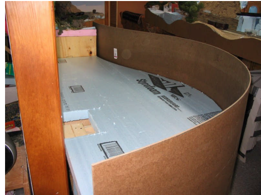
Photo 8 – After cutting, the foam can be put into place. Note the hole cut to clear the radial gusset plate.
