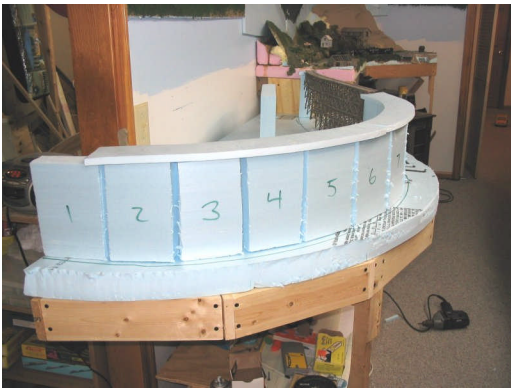
Photo 17 - The ½ inch foam provides a smooth, continuous surface for track roadbed.
