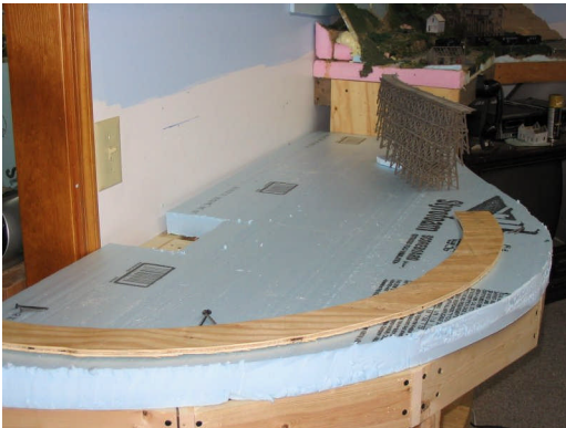
Photo 9 – The fascia is removed to make it easier to work. The trestle is put into location, as is a 24 inch radius template for the curve. These are traced to show the location of the risers on the foam base.
